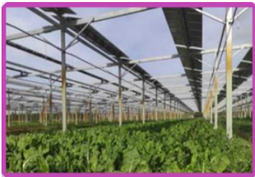
Figure 17 : Ombrières trackers dynamiques (Source : TotalEnergies)
